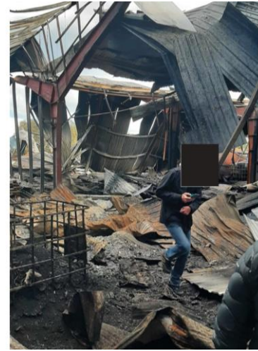
Figure 4 – Extensive fire damage, 2021
