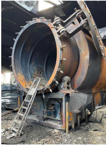
Figure 2 – Reactor endcap torn open, deformed, 2021
