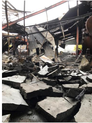
Figure 3 – Walls toppled due to explosion, roof gone, 2021
