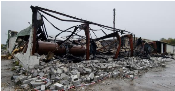
Figure 5 – Walls blown out, 2021
