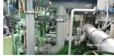
Figure 4: The ship's ballast system
