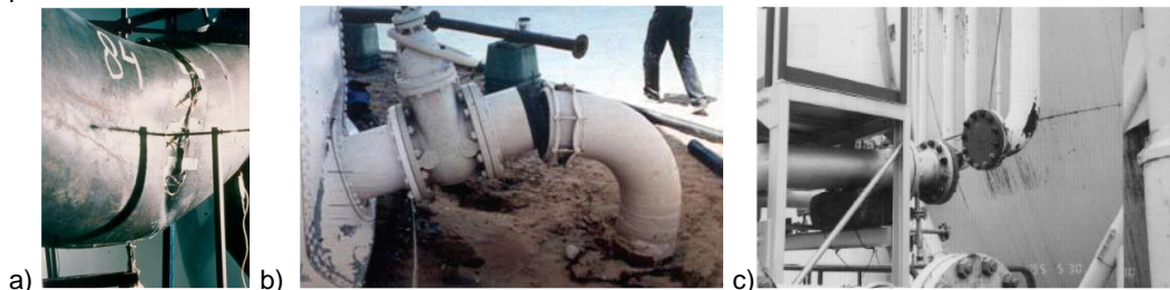
Figure 1: a) local buckling in a pipe (Karamanos et al., 2003), b) failure of the tank to pipe connection (Reza Manshoori, 2011), c) damage on a flanged joint (Paolacci et al., 2012)
